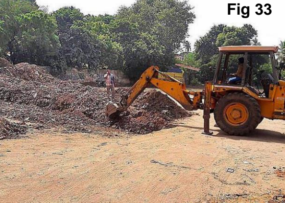
Encroachment of tanks which are neglected to accommodate the rapid urbanisation
